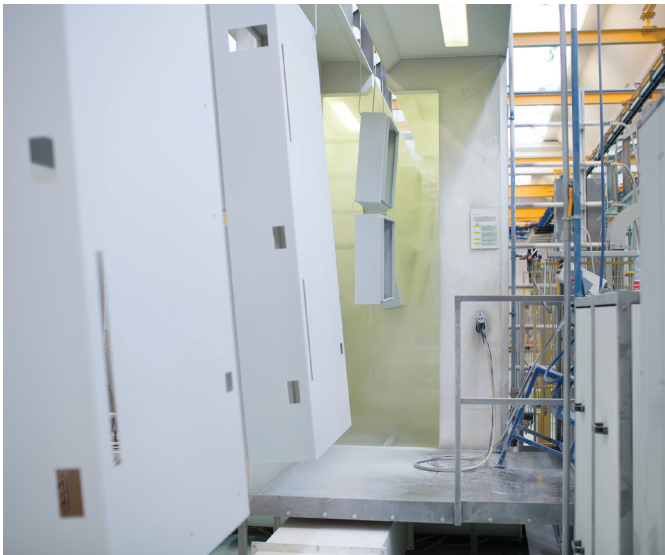
The automated powder coating cabin.
